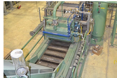
Munitions Treatment Units heat decontaminated munition shells to 1000 degrees Fahrenheit.
