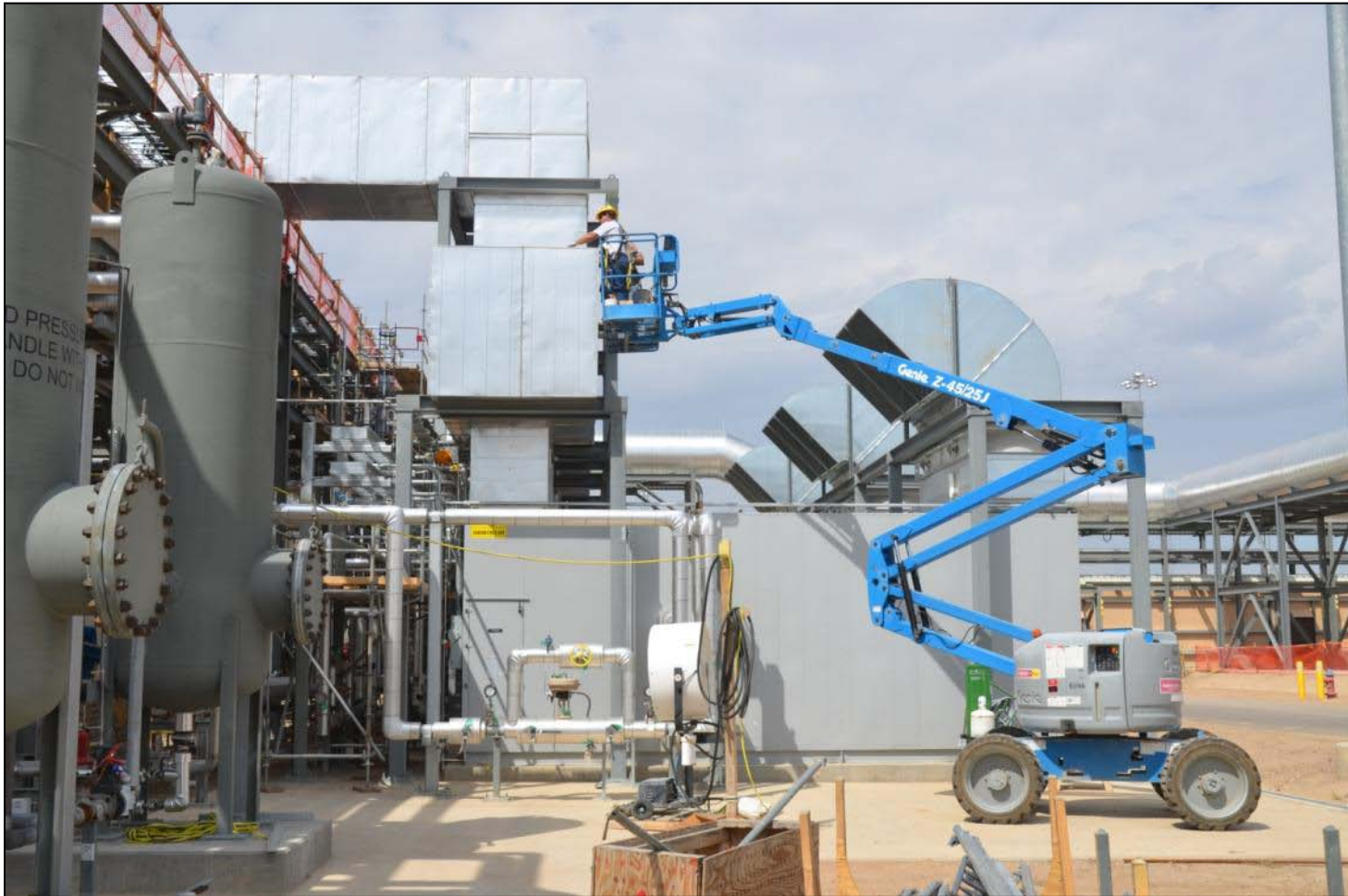
A worker installs lightning protection on the supply air duct of the Agent Processing Building.
