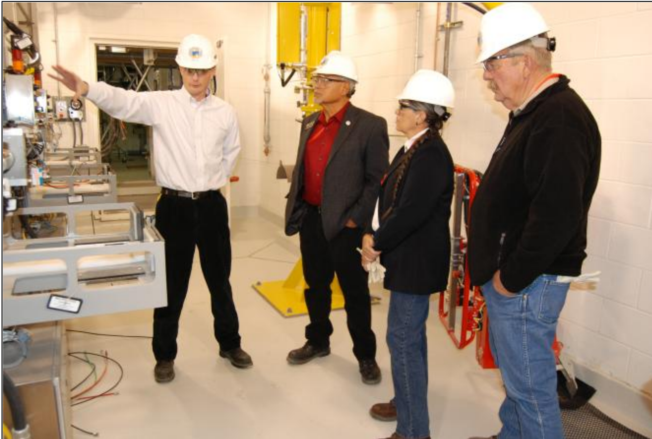
PCAPP Plant Support Manager Dan Hall, points to the Munitions Monitoring Enclosure to explain how munitions are monitored for agent once their energetics have been removed. State Sen. George Rivera, his wife Kathryn, and State Sen. Larry Crowder, toured the site in November.
