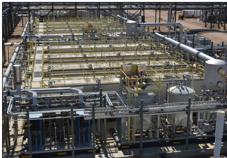
The bioreactors located on the PCAPP site will use common microbes to treat hydrolysate, the wastewater byproduct resulting from the chemical agent neutralization process.
