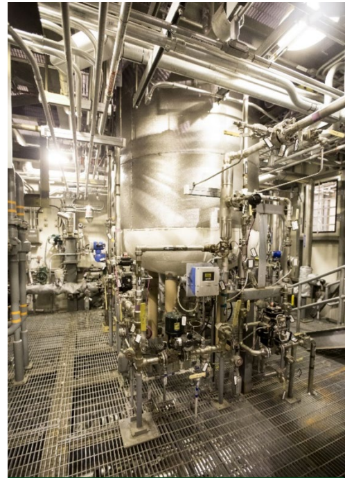
An Agent Neutralization Reactor stands in the Munitions Demilitarization Building at the Blue Grass Chemical Agent-Destruction Pilot Plant. Nerve agent drained from rockets and projectiles is pumped to this reactor and mixed with hot water and sodium hydroxide to neutralize the agent. The resulting product is known as hydrolysate.
