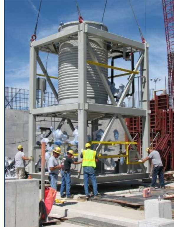
The first two of three ENRs were installed in early September. The ENRs will neutralize explosives that will be removed from munitions.
