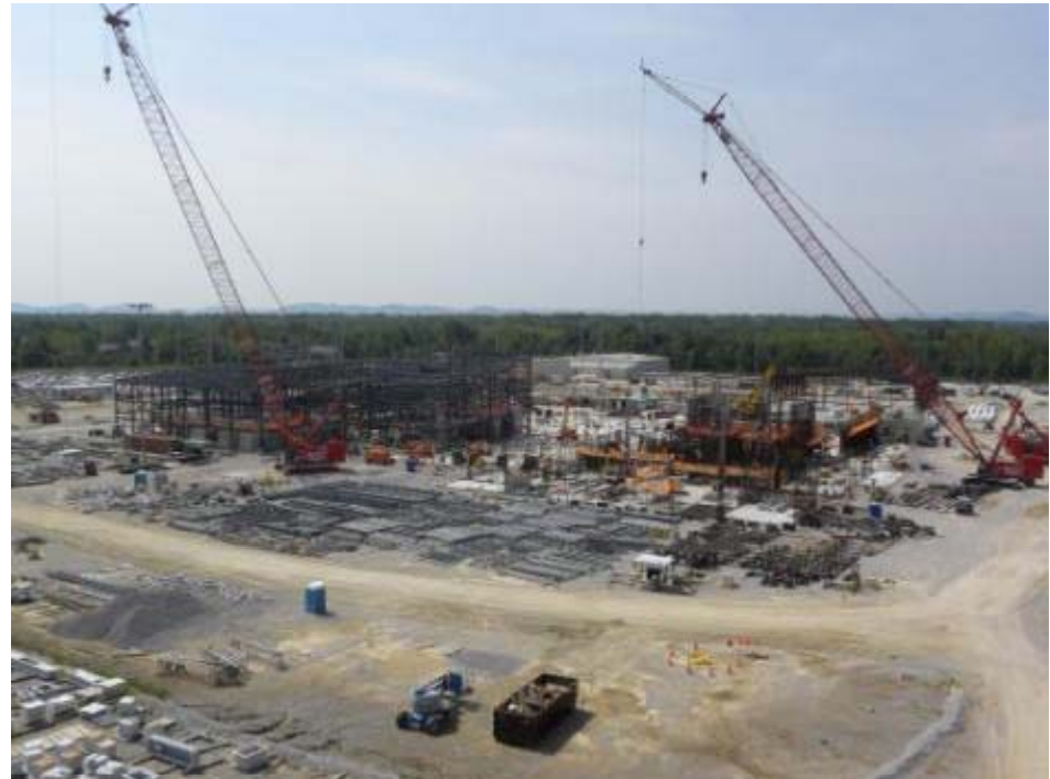
Site photo taken in early July illustrates size and complexity of construction site.
