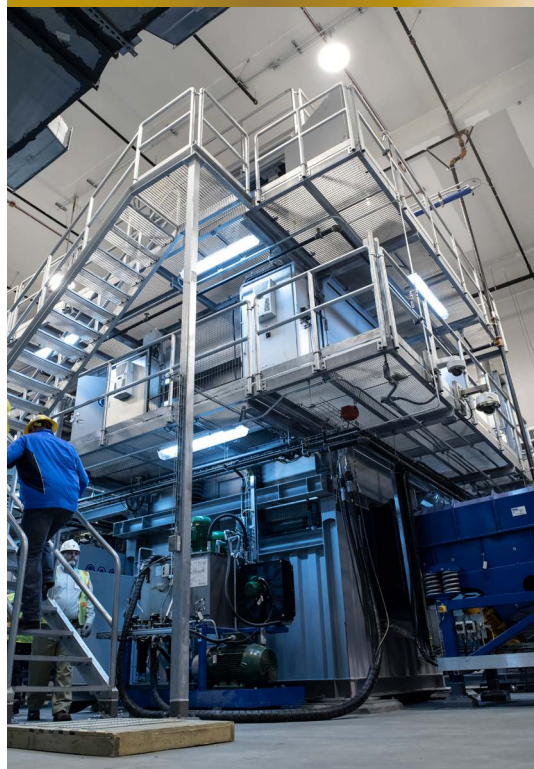
A shift plant manager steps up a staircase next to the Static Detonation Chamber at the Blue Grass Chemical Agent-Destruction Pilot Plant.
